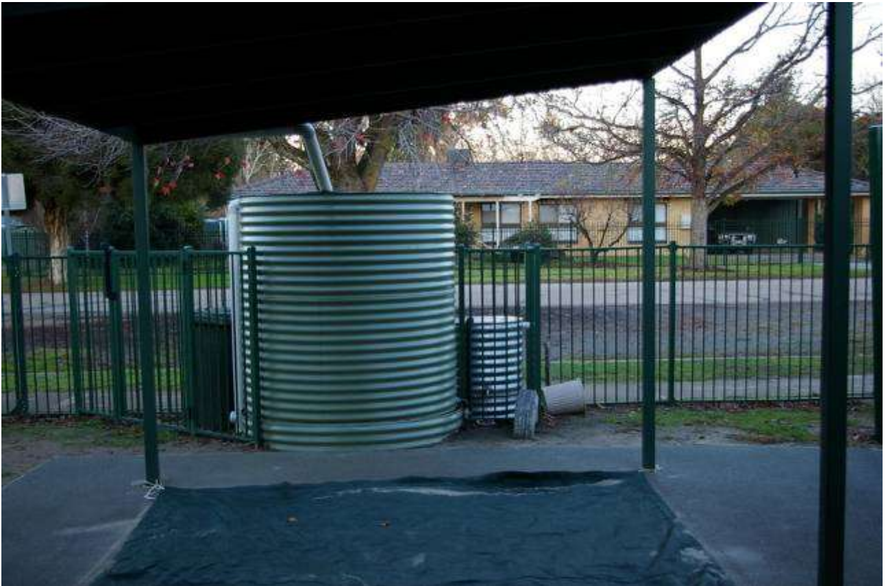
Tanks at early childhood centre. The small tank at right is for the children's use, to fill little buckets for summer play in the sandpit. When it runs out, the children can be
